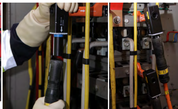
Connection in a power distribution cabinet with Stäubli flat bar clamp
